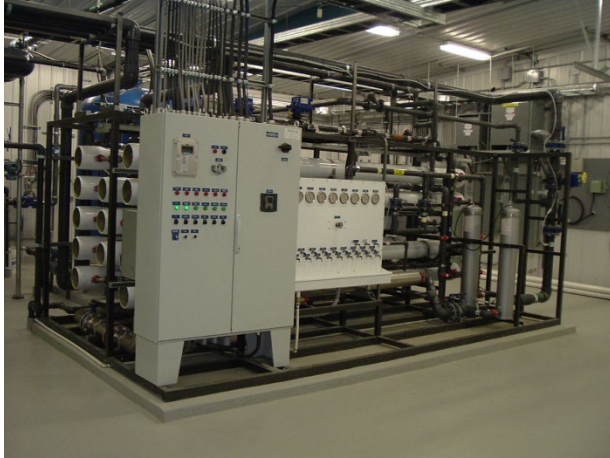
The South RO (original unit)
