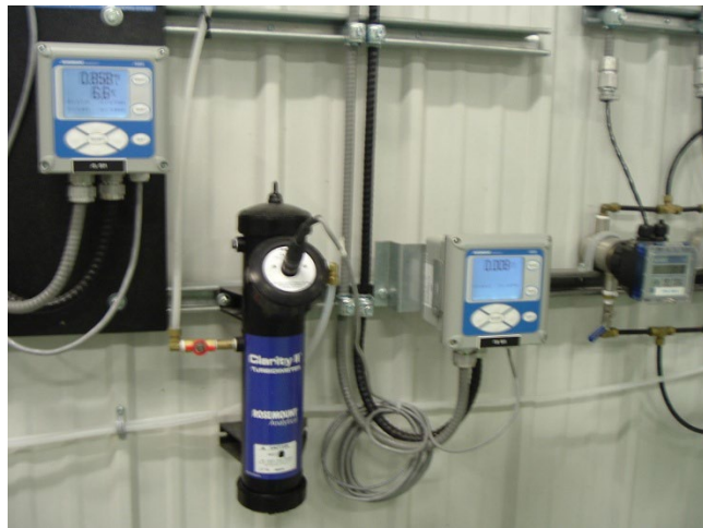
Online Turbidity Monitoring Equipment
