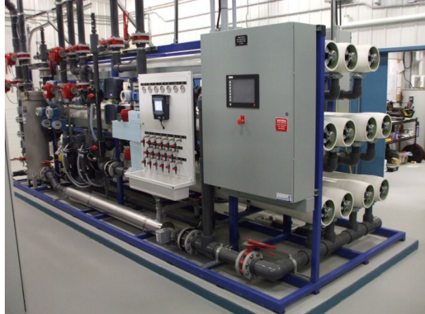
The North RO (new)
